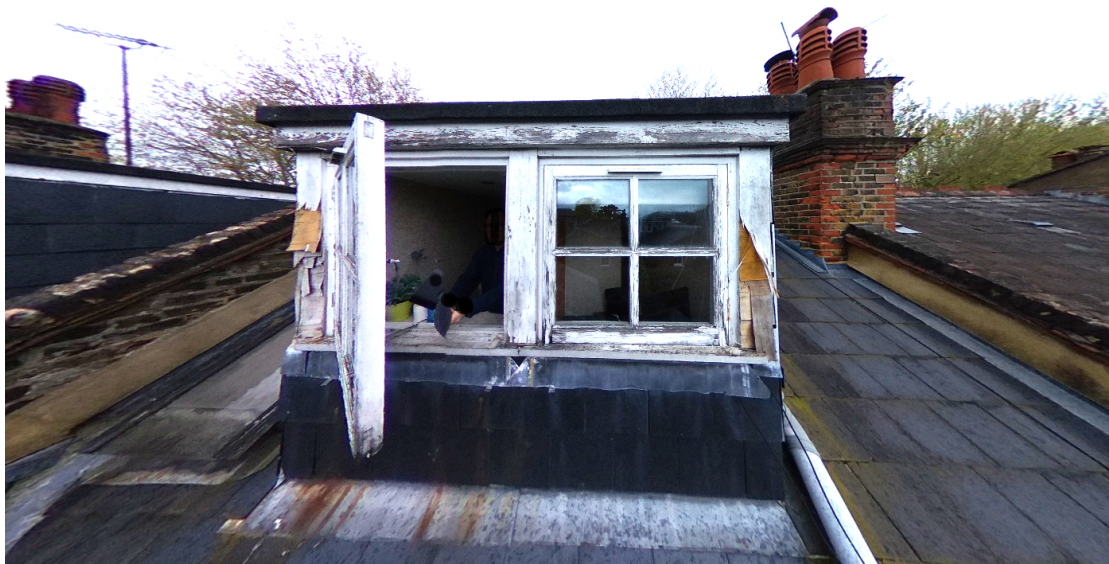
The poor condition of the existing dormer window and stair roof light
