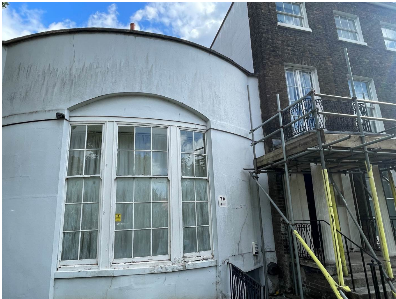
Figure 10, 11 & 12: Existing Timber Window to Flat A
