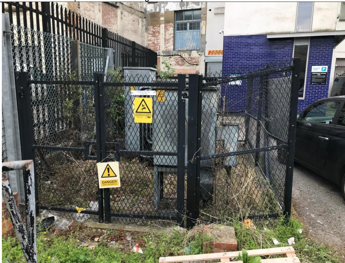
Photo 2: Electrical substation was noted next to the car onsite
