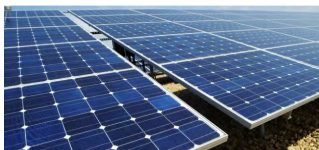
Figure 5: Monocrystalline PV arrays
