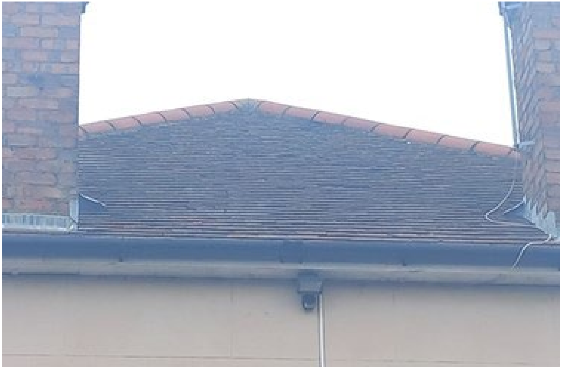
Photo 4 - Building 1 - Tiles and lifted lead flashing
