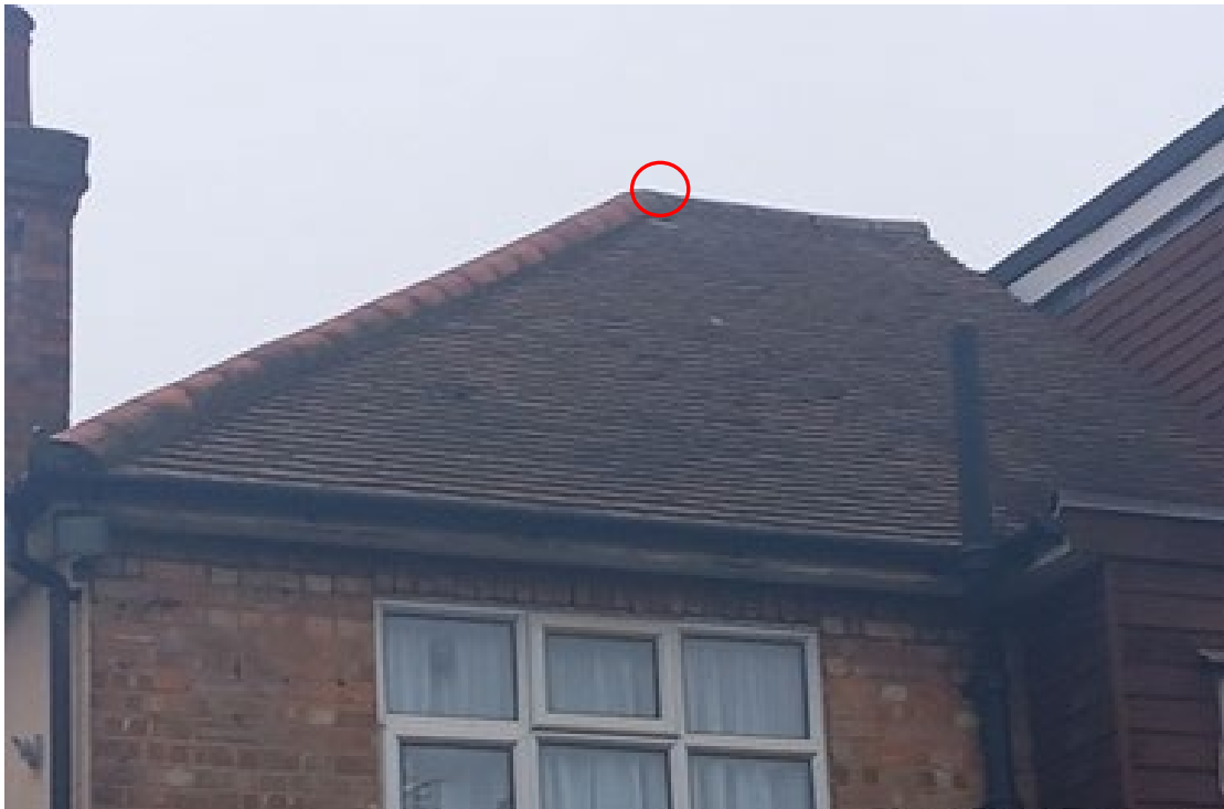
Photo 5 - Building 1 - Rear tiles, including gap
