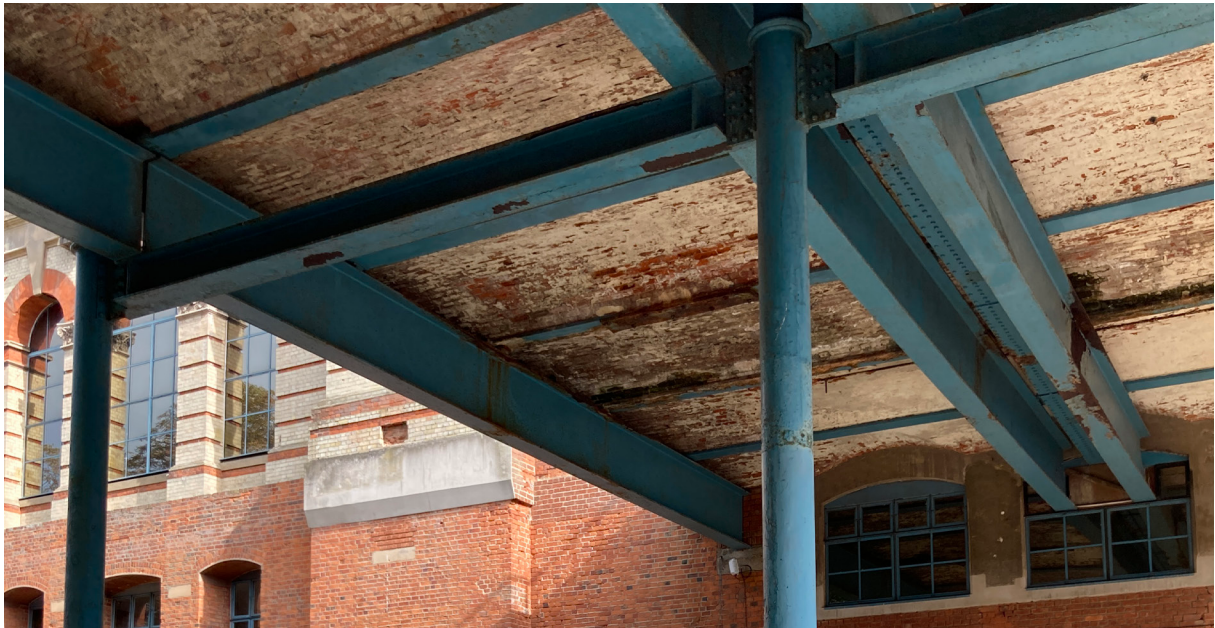
Figure 8: Underside of bridge with visible rusted beams and water ingress through brick vaulted arches
