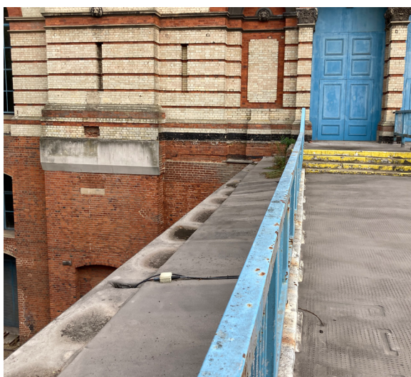
Figure 7: Blistered Asphalt to existing bridge 'gutter'
