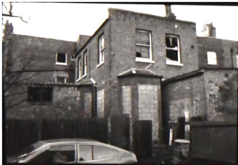
Figure 24 – The rear of Numbers 790 (left) and 792 (right) on 24 November 1977 after the ground floor openings had been blocked up.
