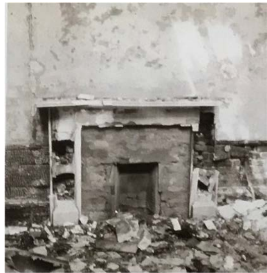
Figure 23 - June 1976 photographs of the fire damage to Number 790
