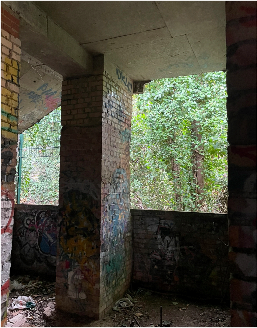
Existing undercroft needs to be secured. Stairs need repairing.
