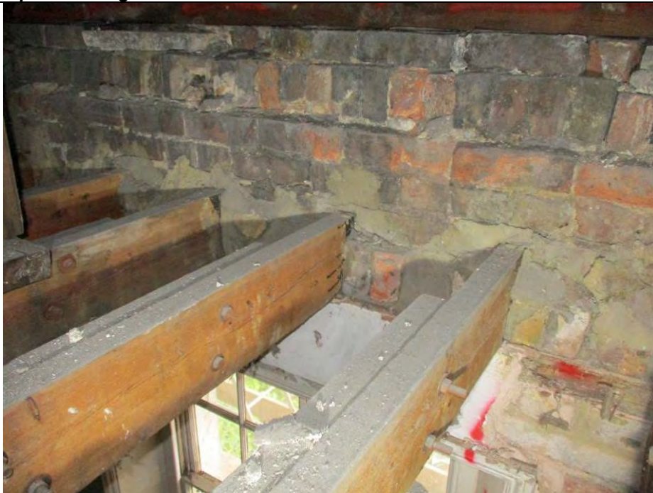
Room S1, showing evidence of previous structural repairs along the east wall. Partnering timbers with bituminous painted ends set in cement mortars are present along east masonry.
