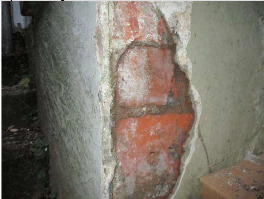
Front elevation, showing damage to render which forms the pilaster detail that has been applied over brickwork. Pilaster render is formed of a cement-based render.
