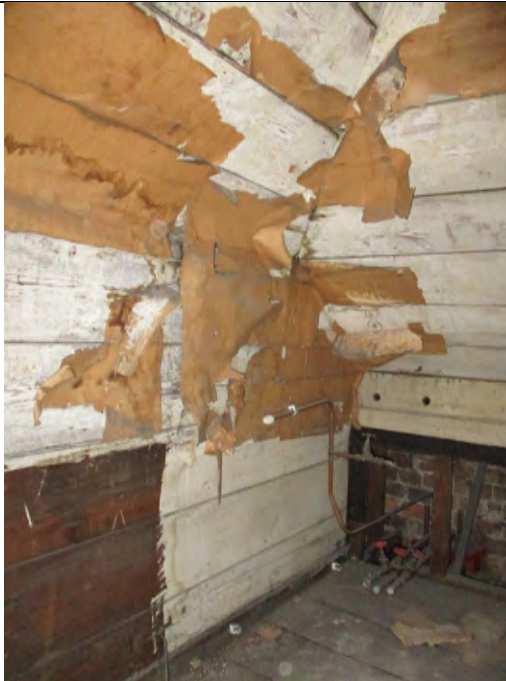
Room S1a, showing interior of cupboard which is lined with horizontal timbers. A lining paper had been stuck over the timbers and is peeling away.
