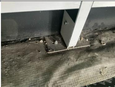
MEC are unable to check the gasket detail to the curtain wall steel bolts.
